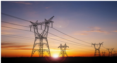
Electric T&D Infrastructure
