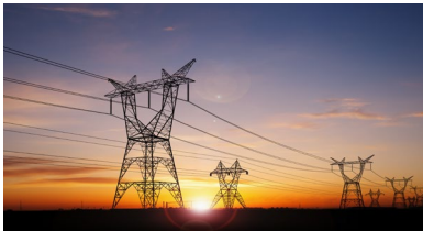
Electric T&D Infrastructure
